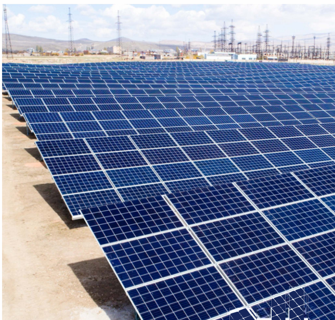
Solar power plant, Talin
